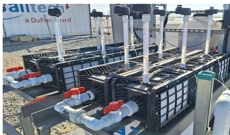
Figure 3. MFC Pilot Skid.
